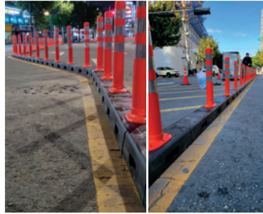
Gusan station - Completed in 2021
